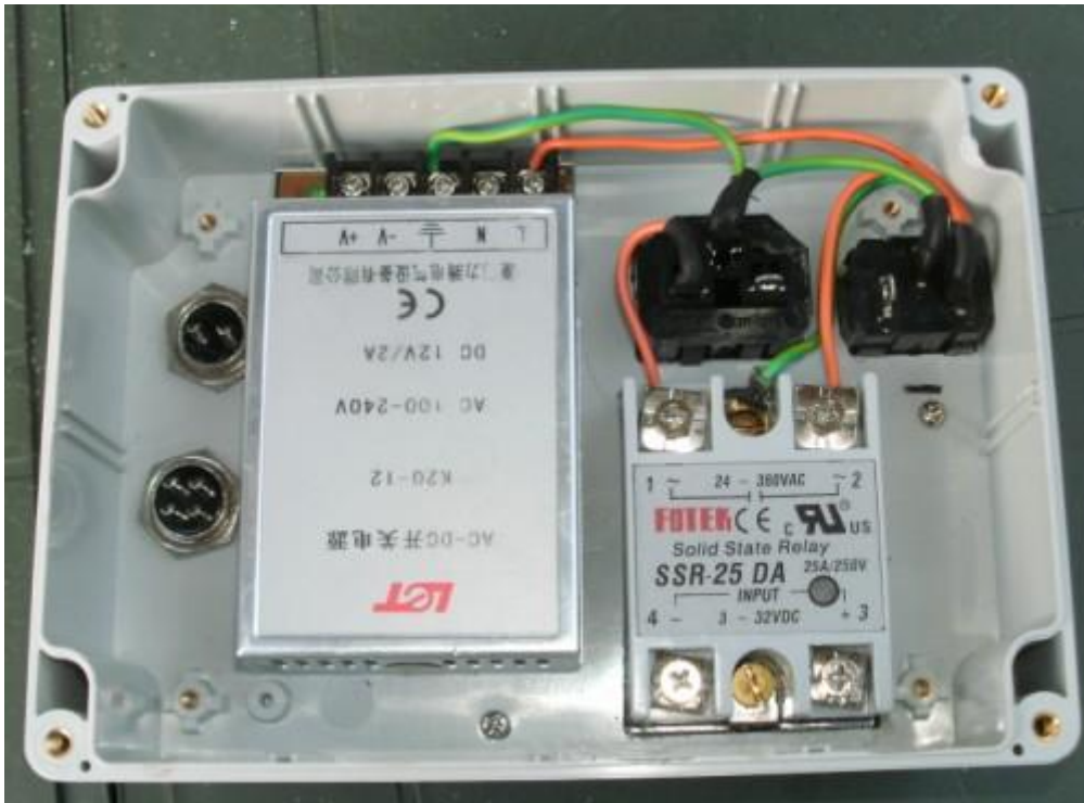
The Active wiring
