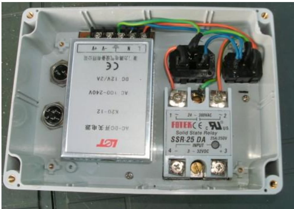
The neutral wiring
