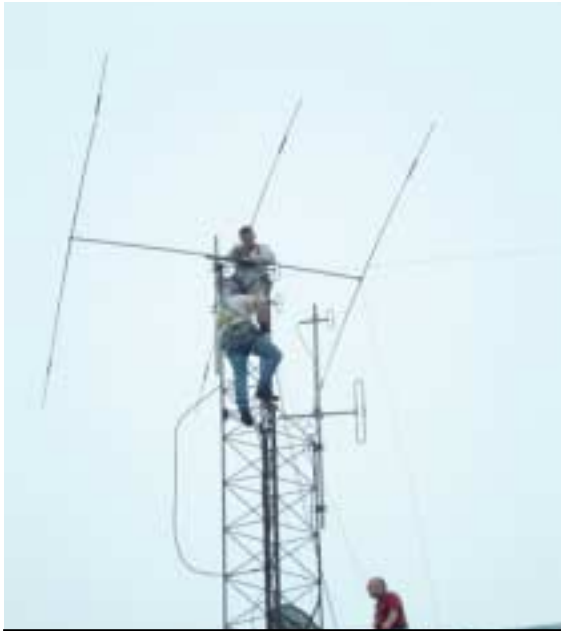
Hams mount additional antennas on the Eric Spicer Building roof during a simulated emergency.
