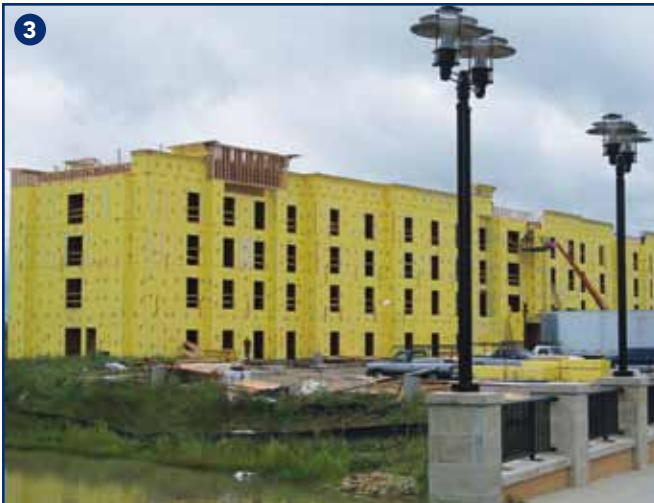
(3) Today's lightweight wood frame structures include large commercial buildings, such as this hotel, which can be enormous and include huge unsprinklered void spaces and potentially include huge unsprinklered void spaces. The entire structure is being wrapped in synthetic foam insulation. (Photo by author.)
